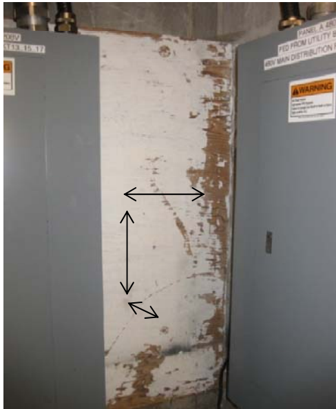
Figure 2.16a: Kiggins Commons distribution panel potential location #1.
