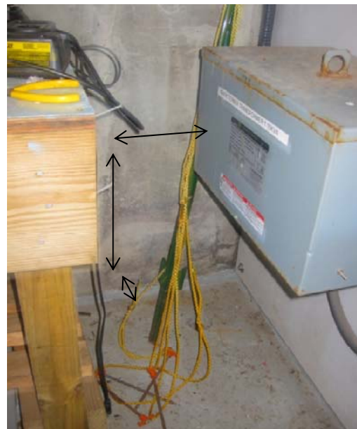
Figure 2.17b: Radar Tower distribution panel potential location #1.
