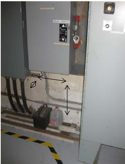
Figure 2.15a: Utility building distribution panel potential location #1.
