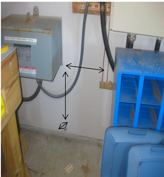
Figure 2.17a: Radar Tower distribution panel potential location #1.
