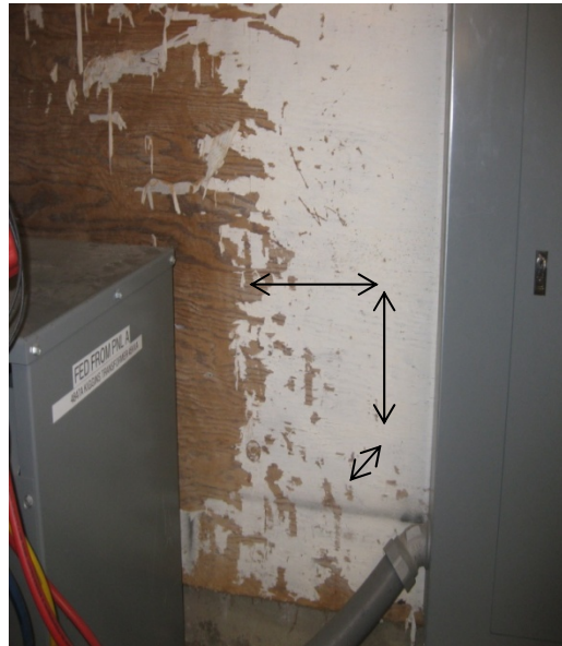
Figure 2.16b: Kiggins Commons distribution panel potential location #2.
