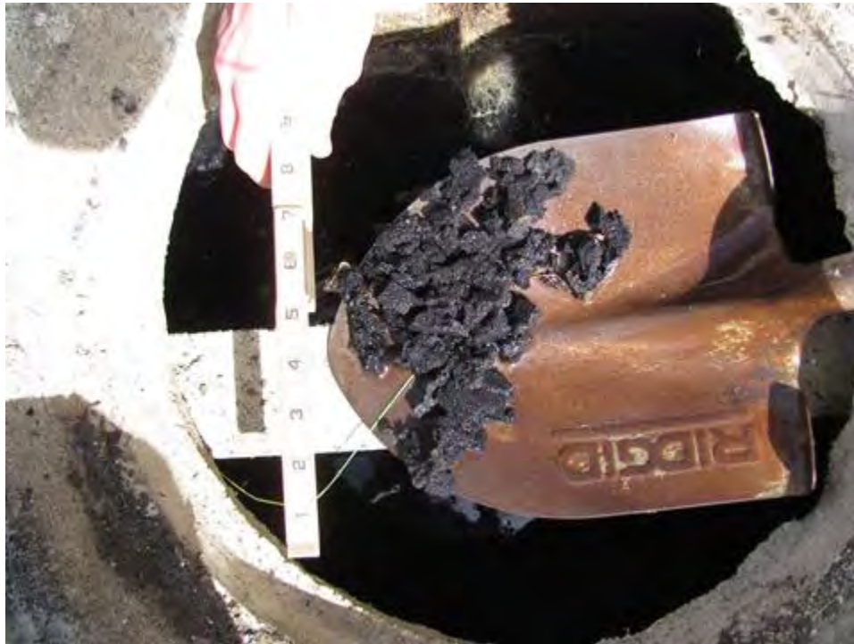
Figure 7.3 - Foam media in section 1 & 2 shows signs of anaerobic activity.
