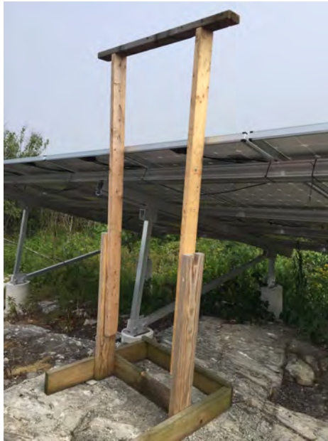
Figure 22: Perch Deterrent System
