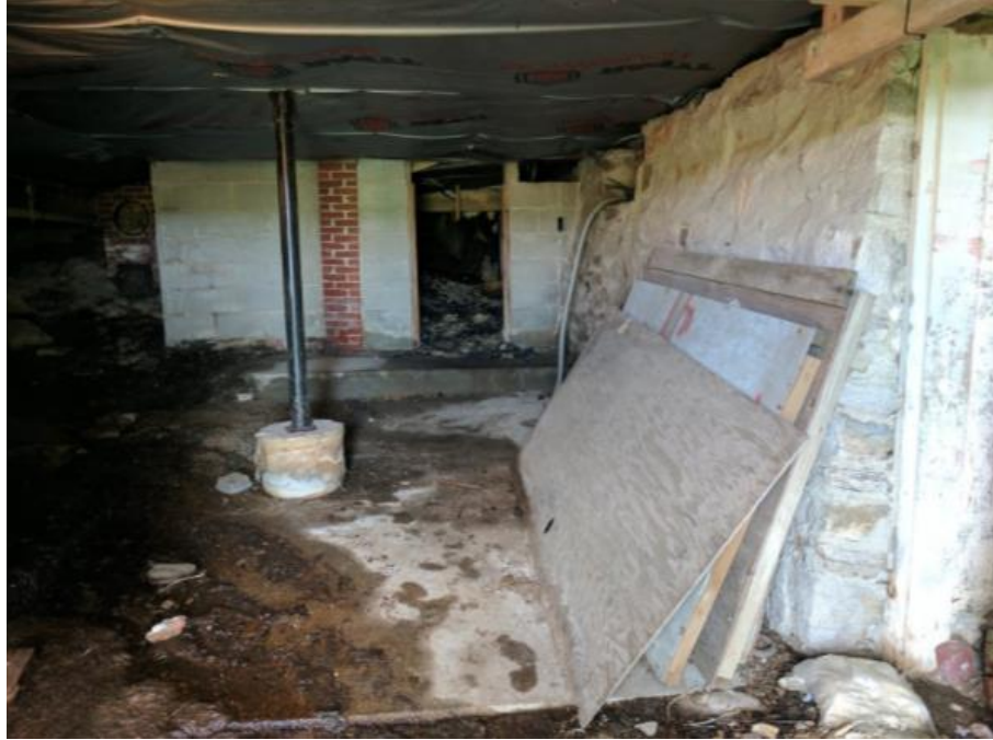
Figure 12. Picture of the basement of Founder’s Hall. To the right of the pole is the concrete slab that could hold water storage tanks
