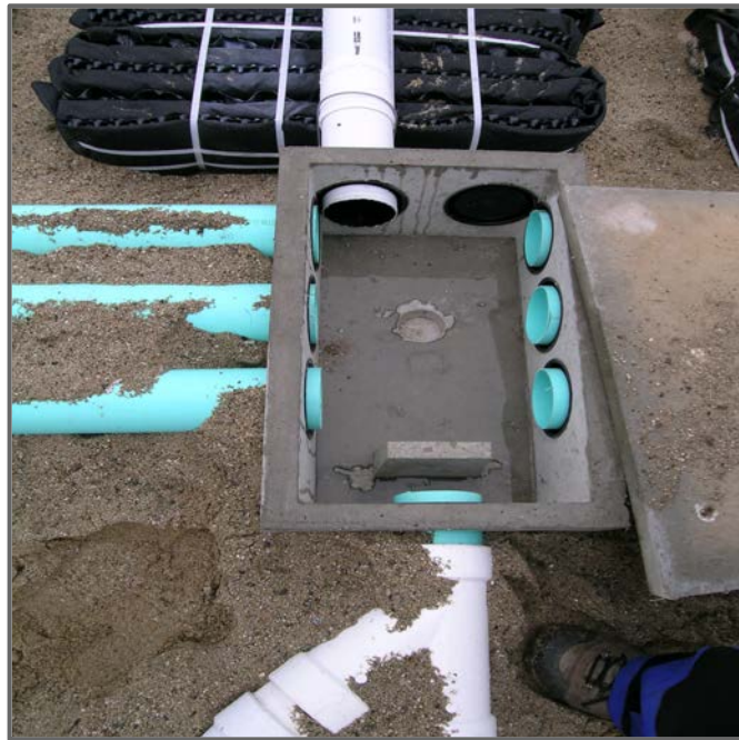
Figure 23: Distribution Box Next to Dorm Septic Tanks
