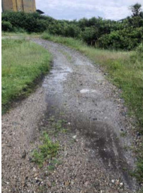
Figure 4.16: Water path during rainstorm, 6/17/2022 at Site 2.
