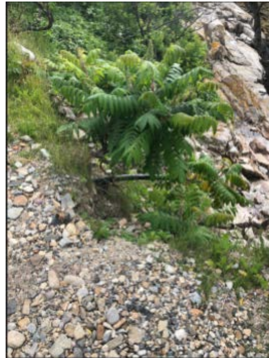
Figure 4.11: Pipe protruding from hillside at severe coastal erosion site 6/16/2022.
