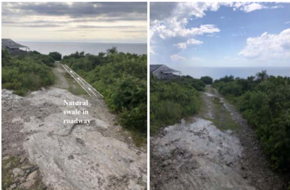
Figure 4.21: The natural swale in the roadway seen on 6/16/2022 and during the rainstorm 6/17/2022. Water flows through the roadway, deepening the swale and increasing the removal of fines.
