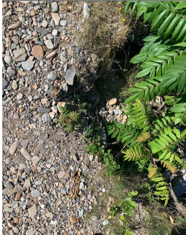
Figure 4.2: Erosion caused by winter storm damage
