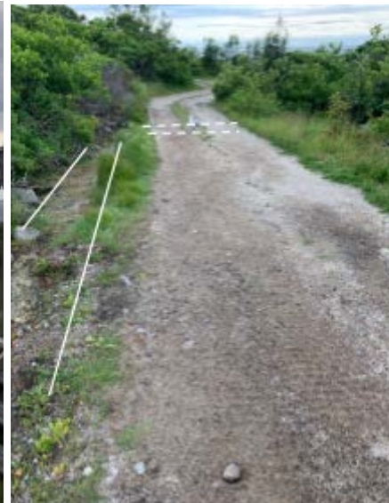
Figure 4.15: Swale and under road drainage, preventing the washing away of fines at Site 2, 6/16/2022.
