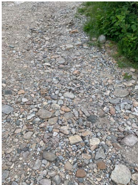
Figure 4.3: An eroded area of road
