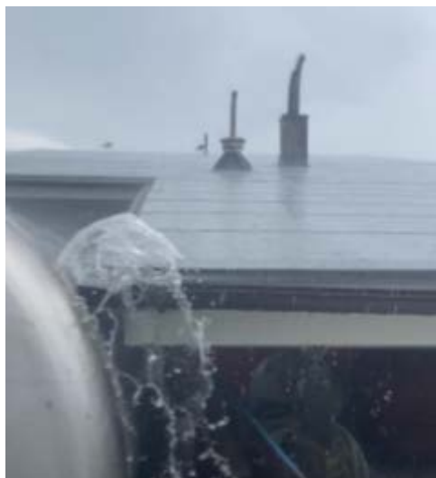
Figure 5.6: Rainwater overflow at Utilities Building gutter, leading to current rainwater storage tanks
