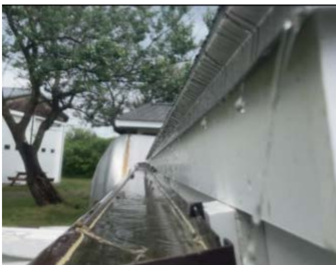
Figure 5.7: Utilities Building gutter during rainstorm; note the water dripping between the edge of the roof and the building
