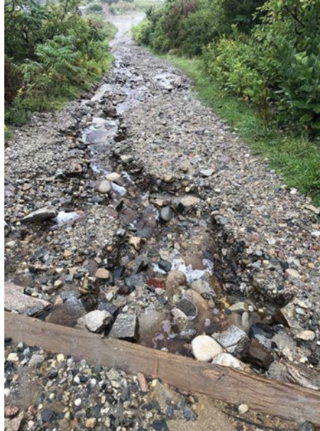
Figure 4.1: Erosion after storm surge
